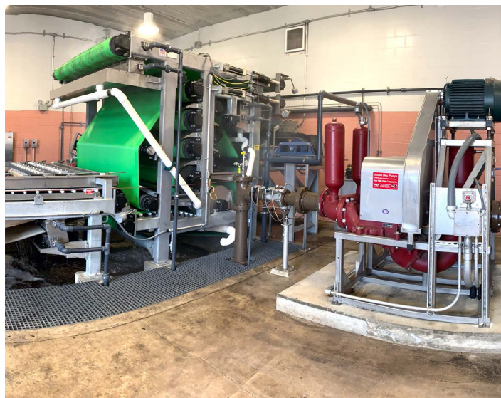
Pictured above is a belt press feed in Florida.
